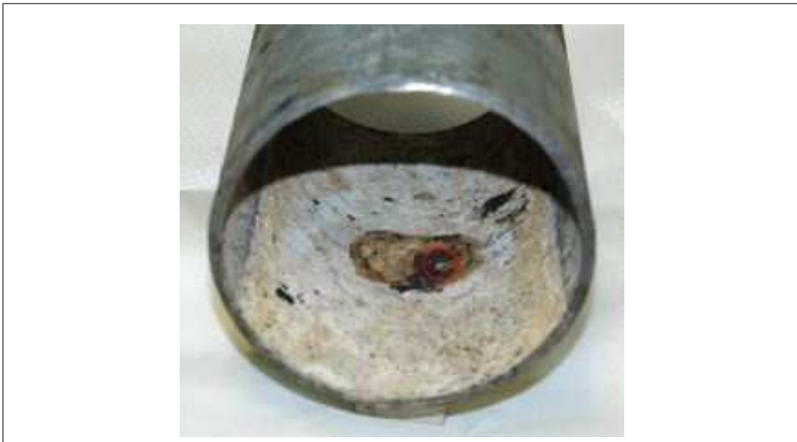
Fig. 9b. Corrosion at the base of a tubercle, which ultimately led to through-wall leakage
