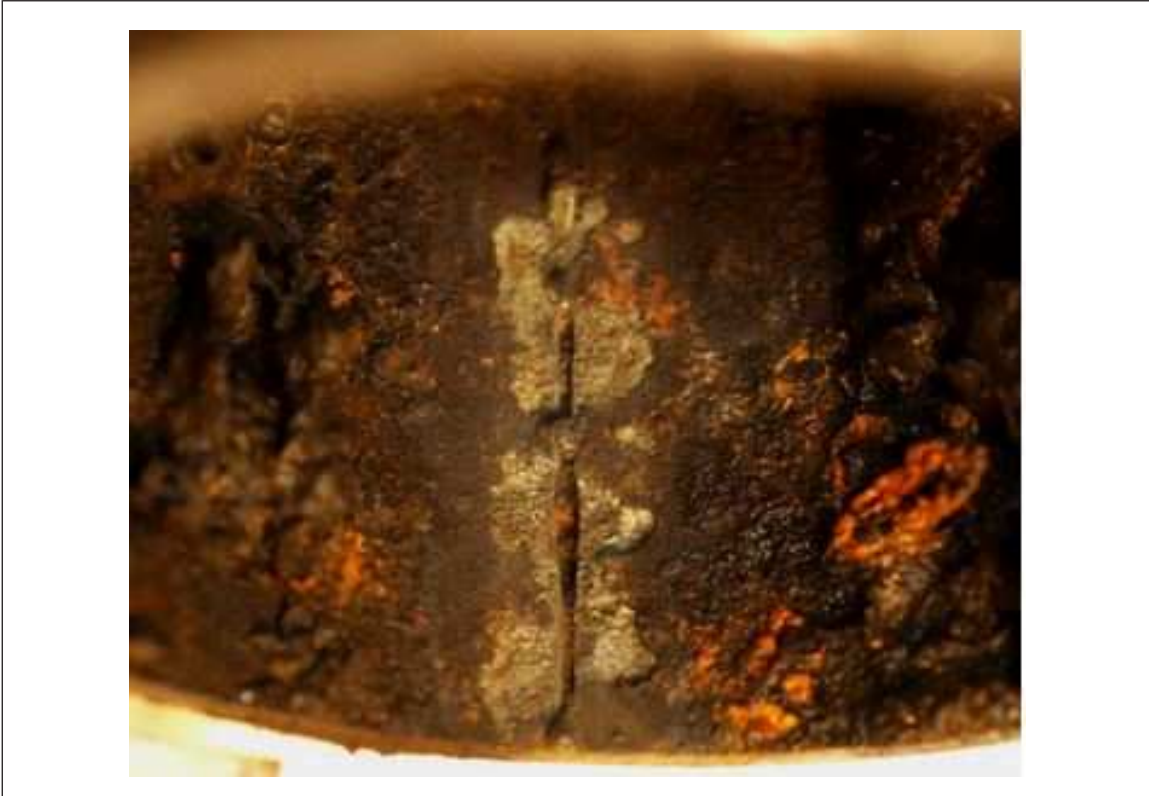
Fig. 11b. Leakage on an NPS 2½ steel sprinkler pipe in a wet pipe system after removal of corrosion products; preferential attack surrounding the weld seam is severe
