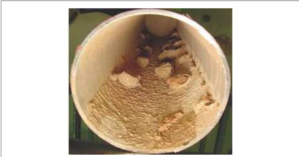
Fig. 9a. Tubercles that formed inside a galvanized steel sprinkler pipe (4 in. [10 cm] diameter)
