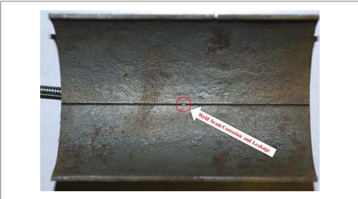
Fig. 12. Preferential grooving corrosion on a pipe weld seam with a .04 in. (1 mm) pinhole leak in a wet pipe system, after removing corrosion products inside an NPS 3 pipe
